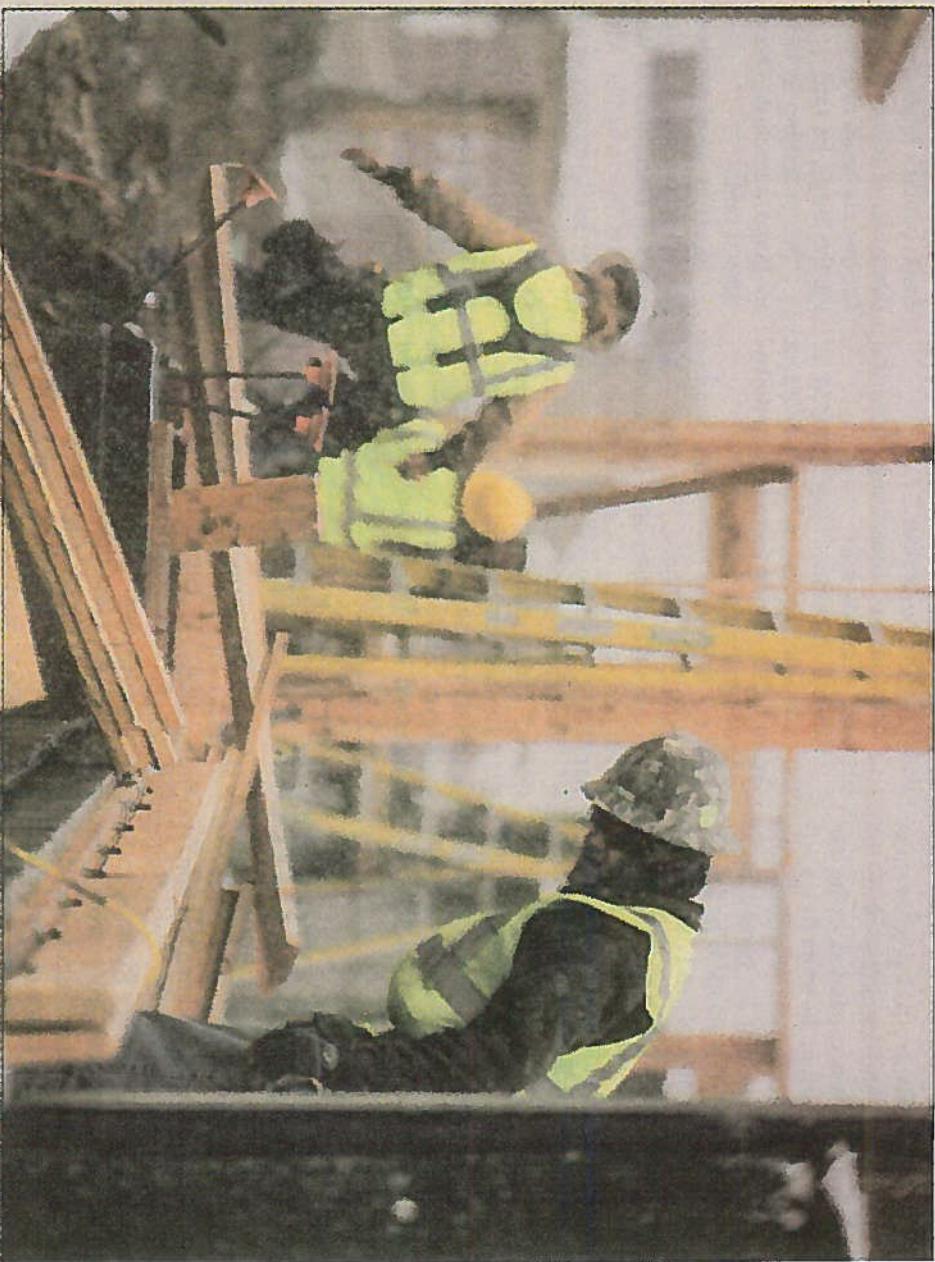
Construction continues in the next phase of Burlingame Ranch, a city affordable housing project that is funded primarily by real estate transfer taxes.
