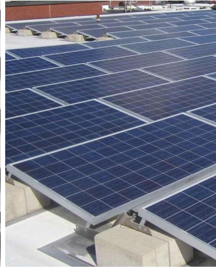
BALLASTED SOLAR PANELS
